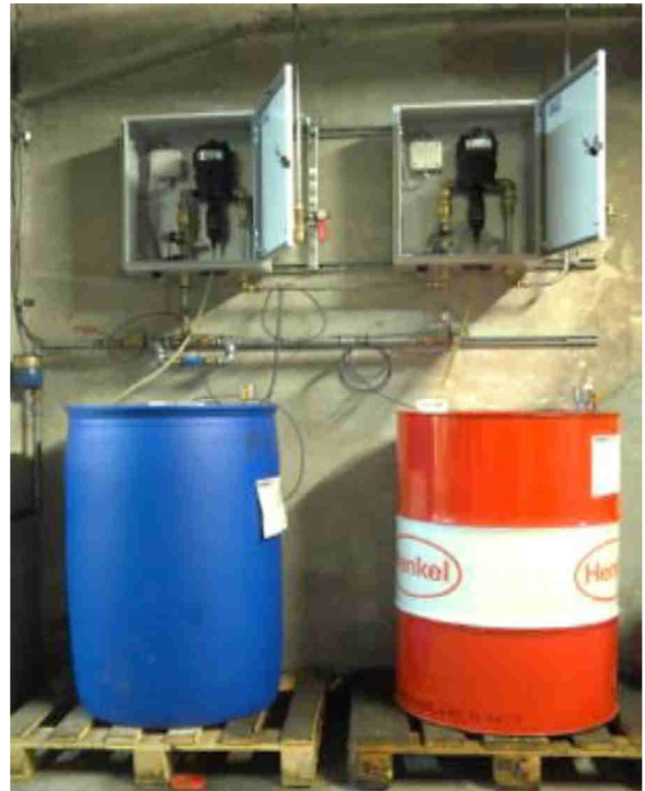
The mixing station provides constant mixing ratios between the two components of the cooling lubricant that are used.
